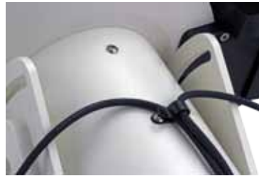
Installed Cable Clip
